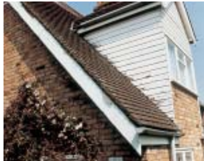
Problem: Decaying timber cladding
